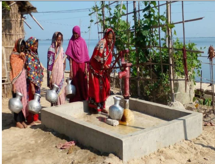
A Deep Tubewell was installed by the project in a flood affected village in Jamalganj, Sumanganj
